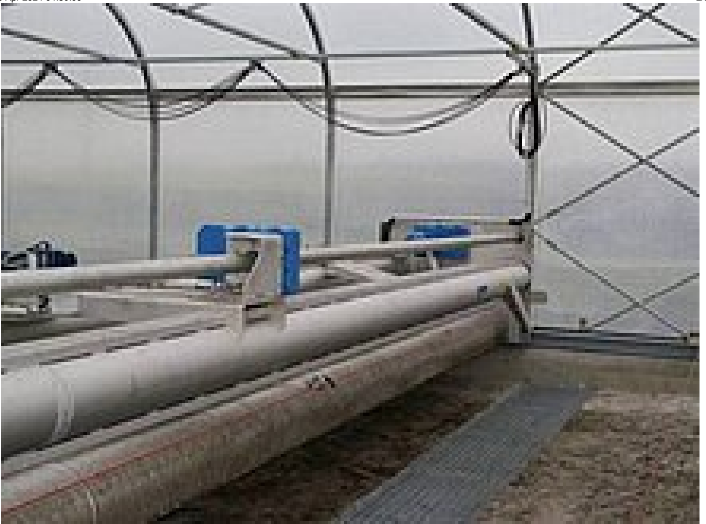
On its way back the sludge turner can drop the dry sludge into a screw that is installed below ground level.
