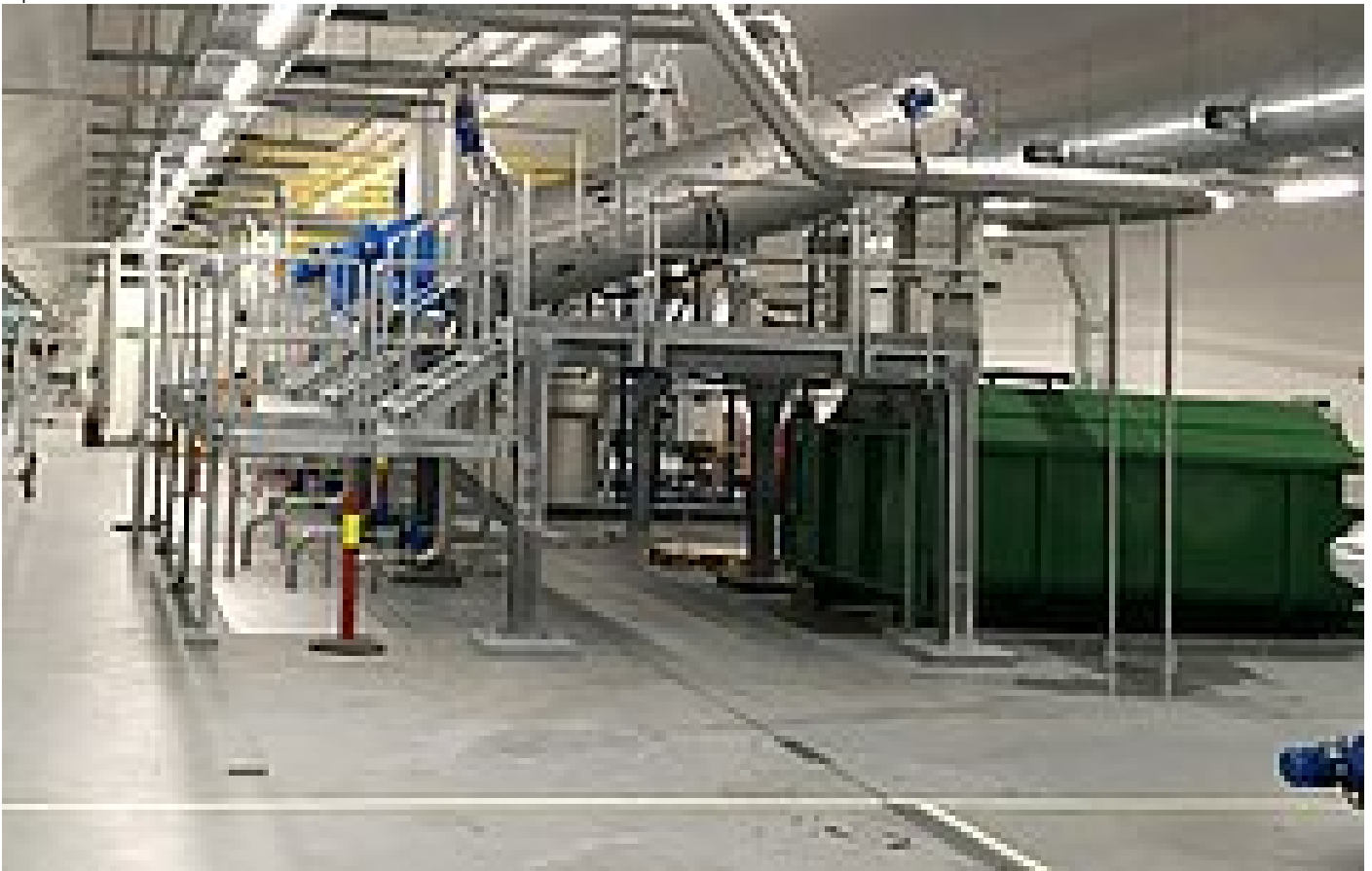
Sludge dewatering with two HUBER Screw Press S-PRESS
