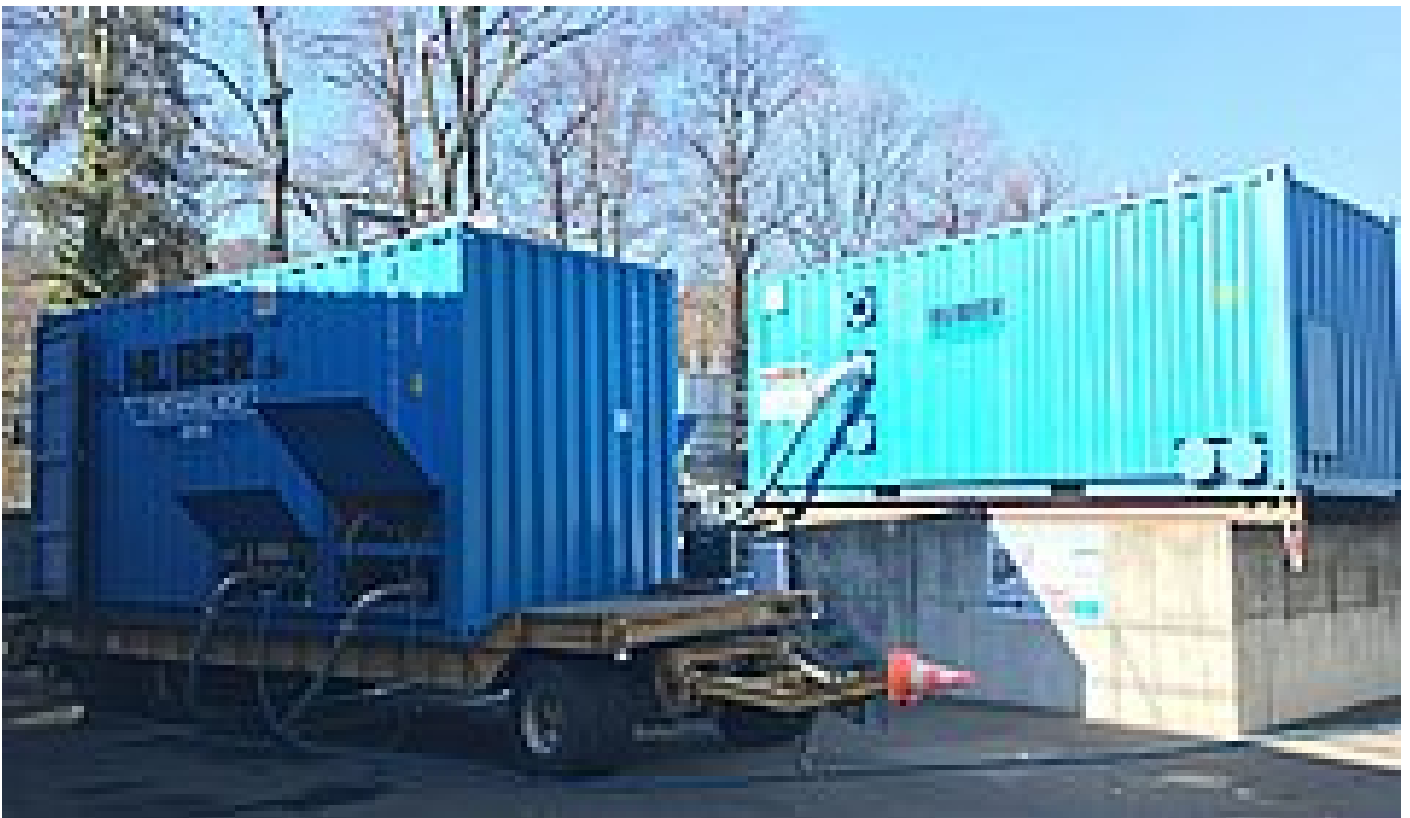
Fig. 4 Validation operation - HUBER Drum Screen LIQUID demo unit (right container) combined with the HUBER Screw Press Q-PRESS® demo unit (left container)
