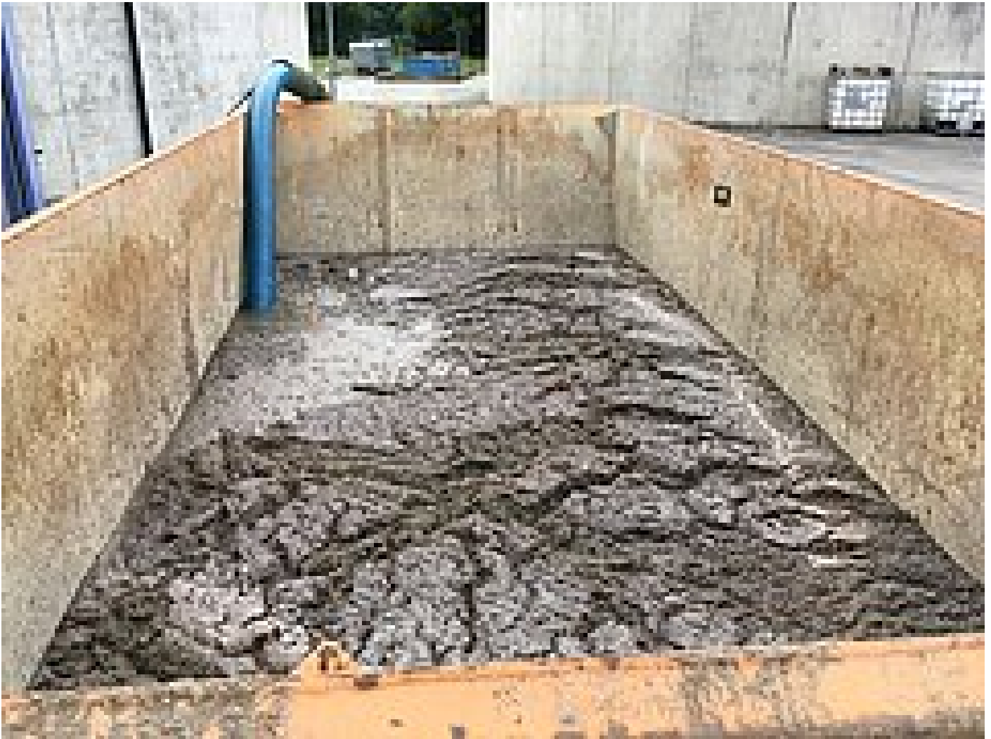
Fig. 3: Thickened primary sludge from the HUBER Drum Screen LIQUID demo unit after a HUBER Disc Thickener S-DISC
