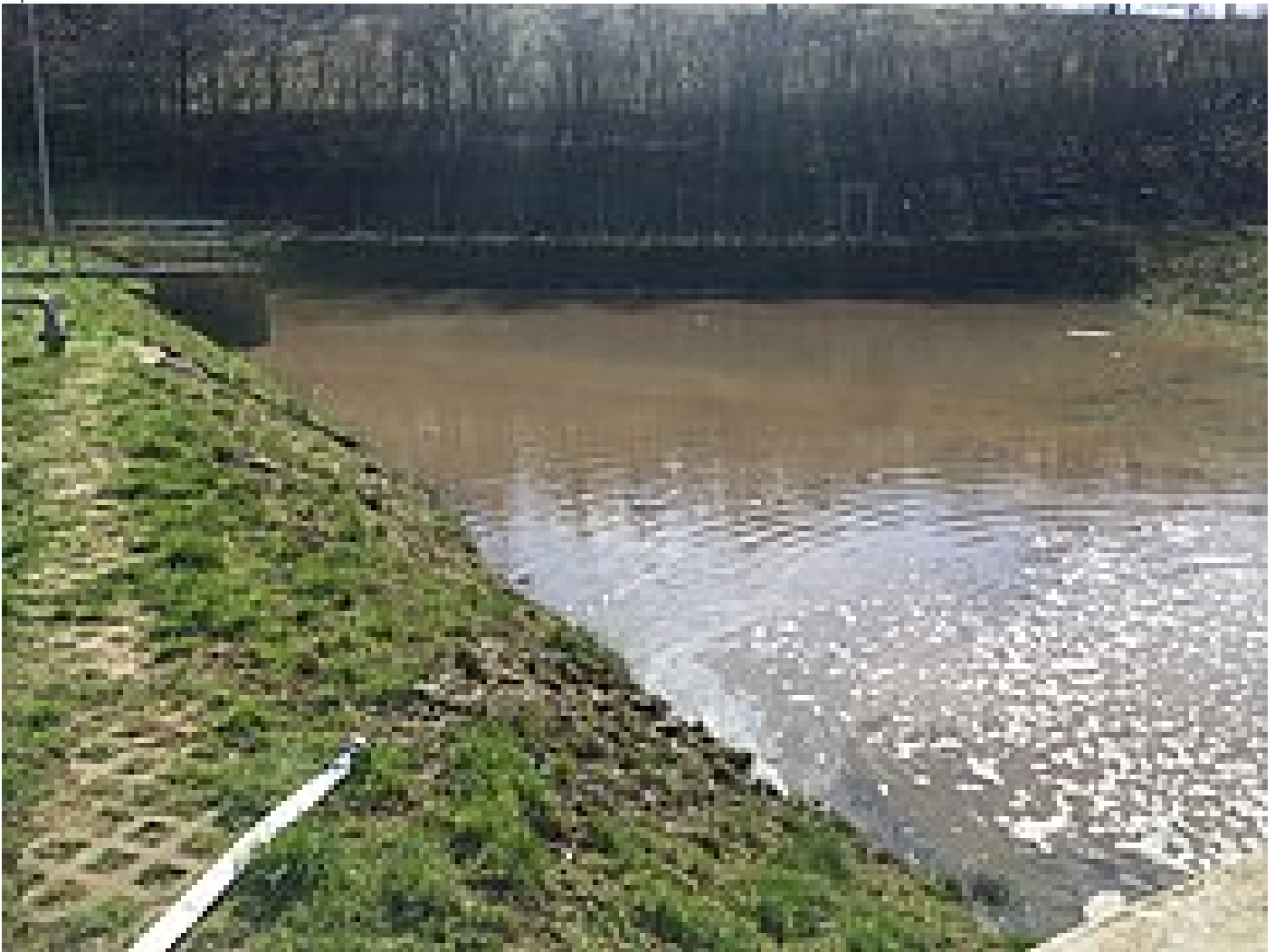
Fig. 6: Bridging operation - polishing pond converted into a settling pond for static thickening of the thin sludge from the HUBER Drum Screen LIQUID demonstration plant
