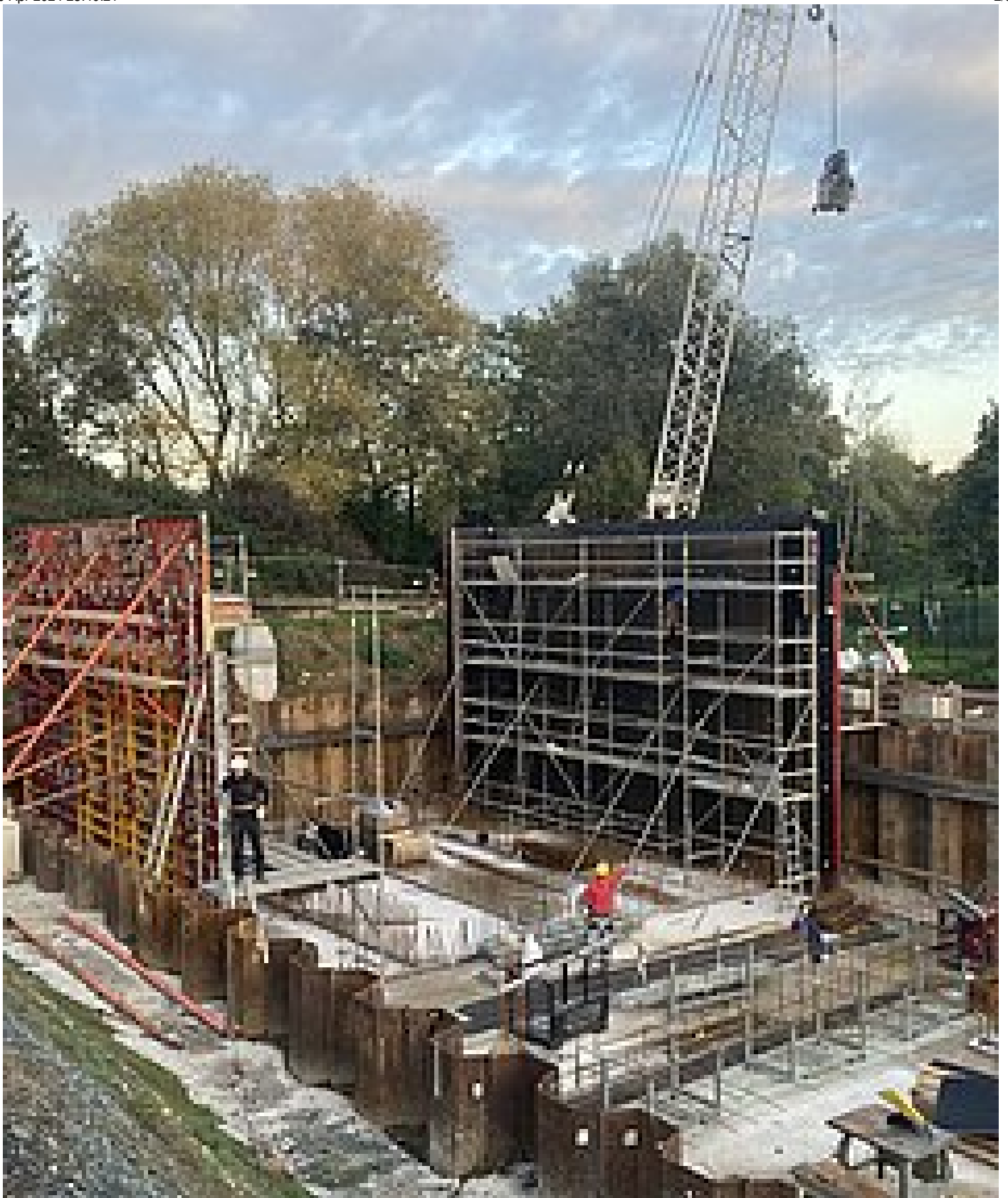
Construction of the activated carbon filter stage in Bickenbach is progressing. (Photo: Jörg Stanzel, Wastewater Association Bickenbach)
