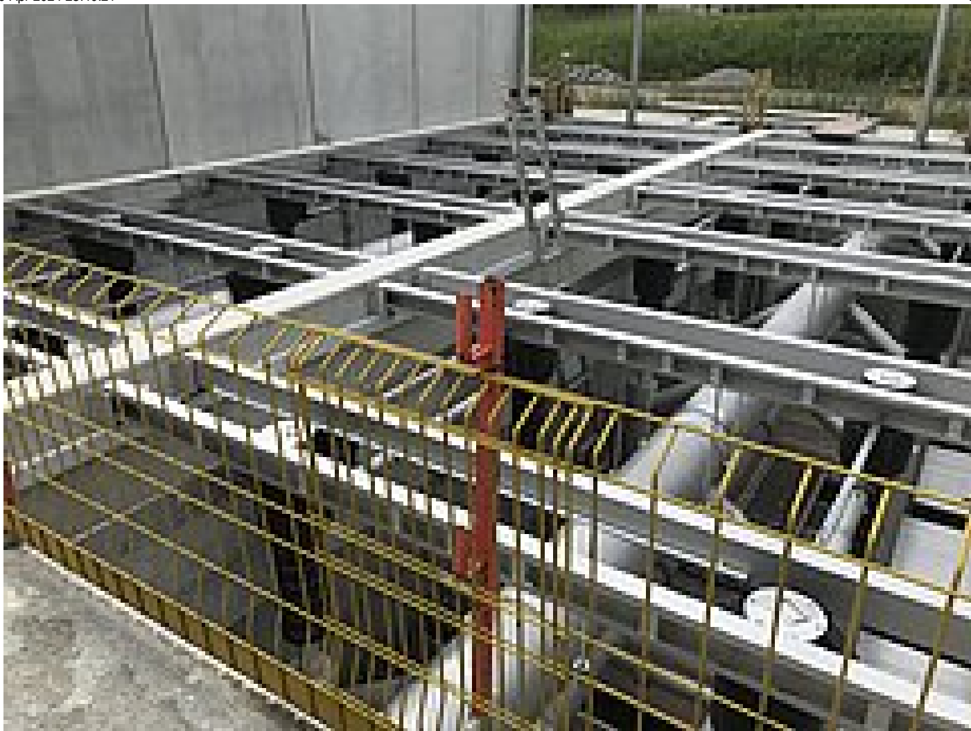
In Uhdingen, the 24 HUBER Activated Carbon Filter CONTIFLOW® GAK units were already installed in summer.
