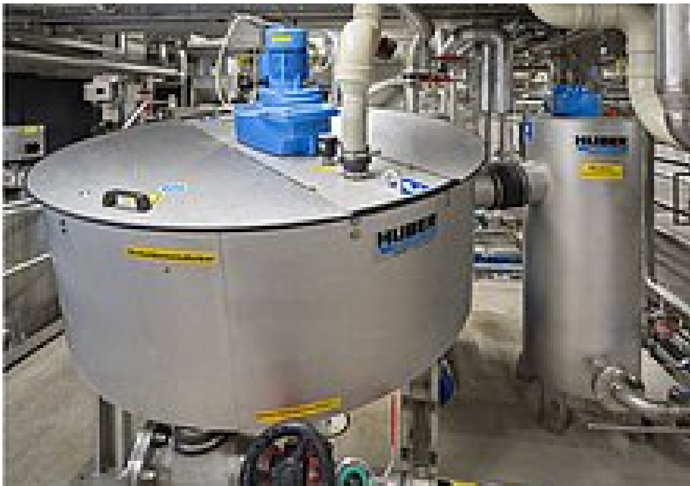
Fig. 5: Thickening of flotata and excess sludge with a HUBER Disc Thickener S-DISC
